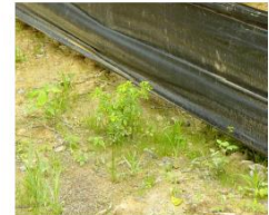
This silt fence was not installed correctly and will not function. It should be "trenched" in to prevent sediment from washing under it. The time spent installing it incorrectly is wasted time. It will need to be reinstalled correctly.
